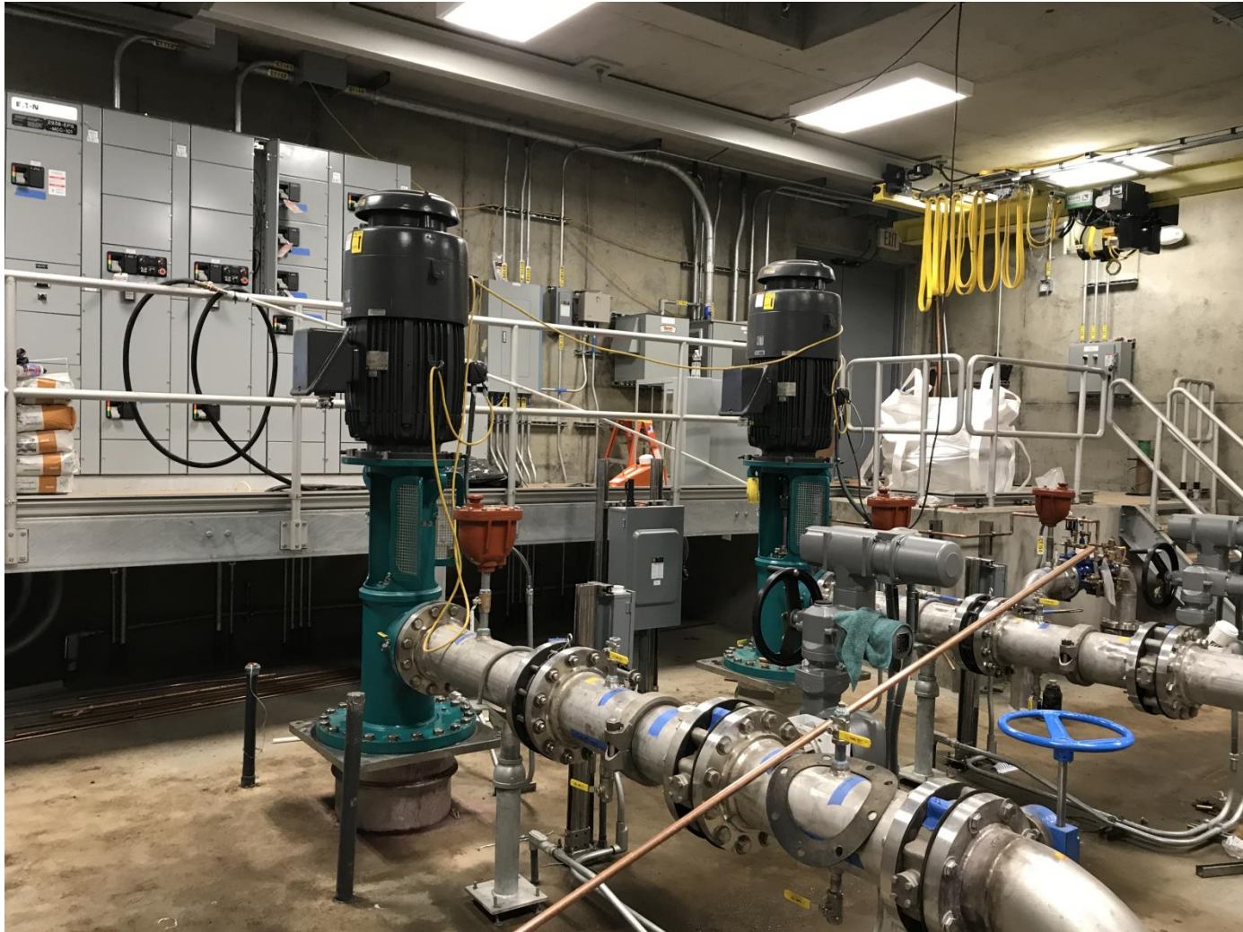
Bayfair Pumping Plant
